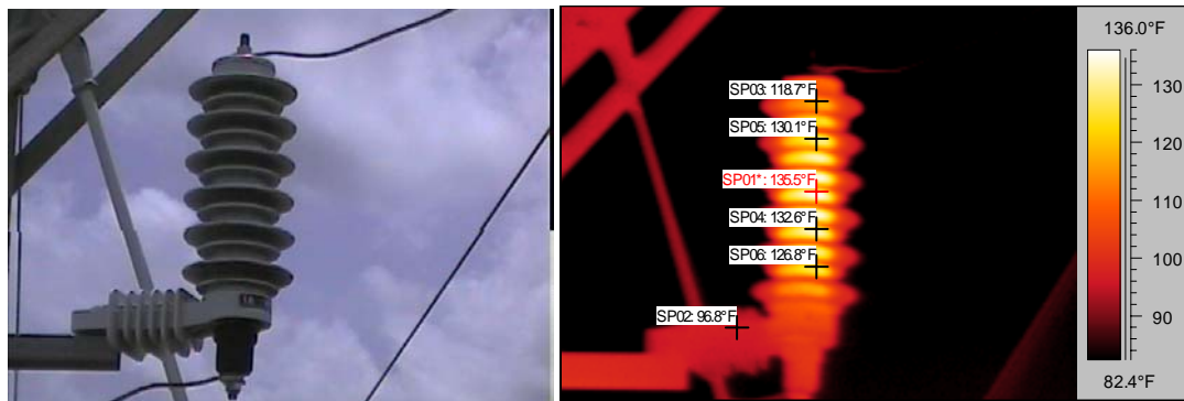
Figure 4. The infrared thermogram shows a high amount of heat present within the arrester, thus causing the feeder to relay open. This also holds true for fused taps. The next page shows examples of the tests on returned lightning arresters that showed un hot on the distribution lines.
