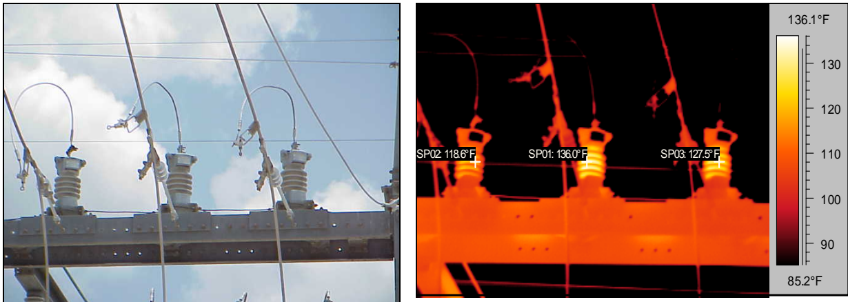
Figure 2. The heating problem with these arresters could have affected the reliability of this three phase feeder line. Feeder lines such as these serve 2,550 consumers.
